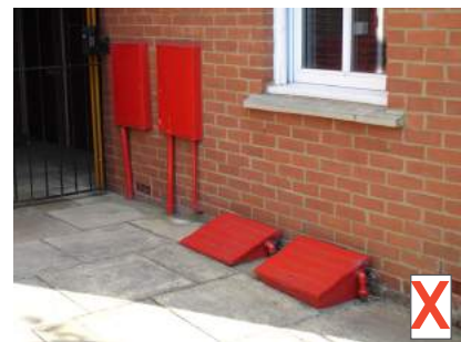
OBTRUSIVE SERVICES BOXES ON THE FRONT OF A HOUSE
