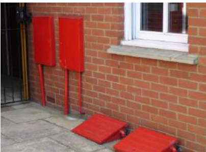
VISIBLE SERVICES BOXES
